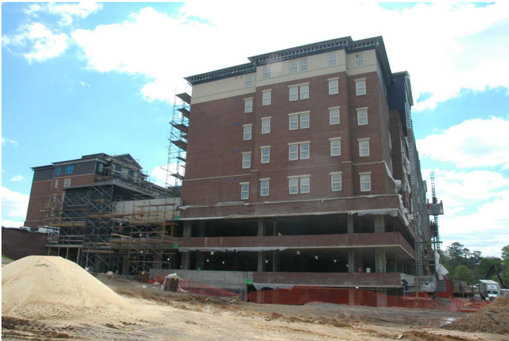
Figure 2 – North Elevation Showing Three Lower Parking Levels and Five Upper Residential Levels
