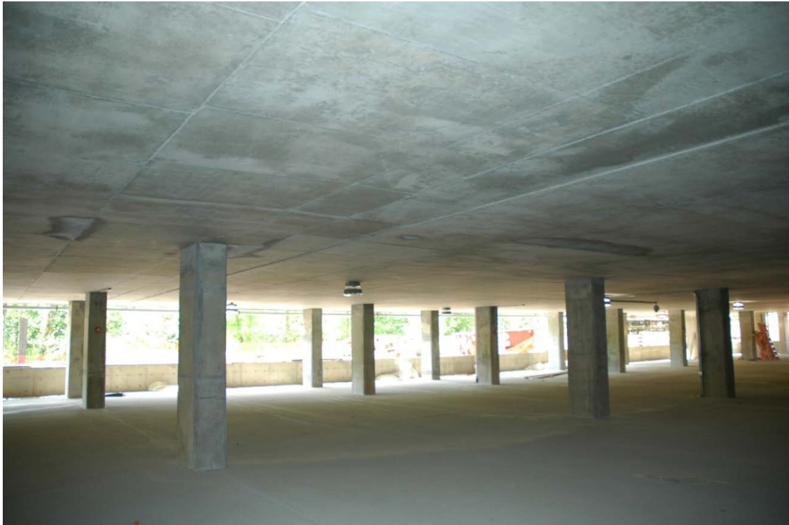
Figure 4 – Soffit of First Level Slab (Standing on Slab-on-Ground) Looking West and North
