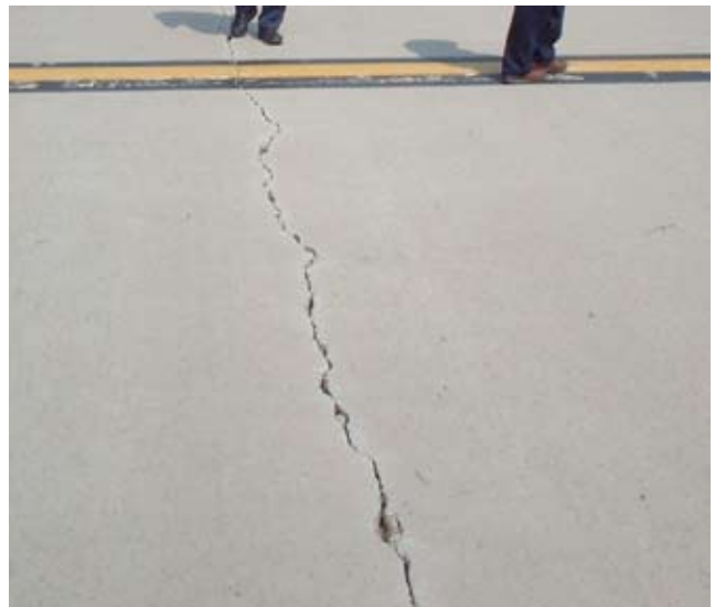
Below: Spalling is evident in this 2003 photo of a crack in the conventional portland cement concrete slab.
