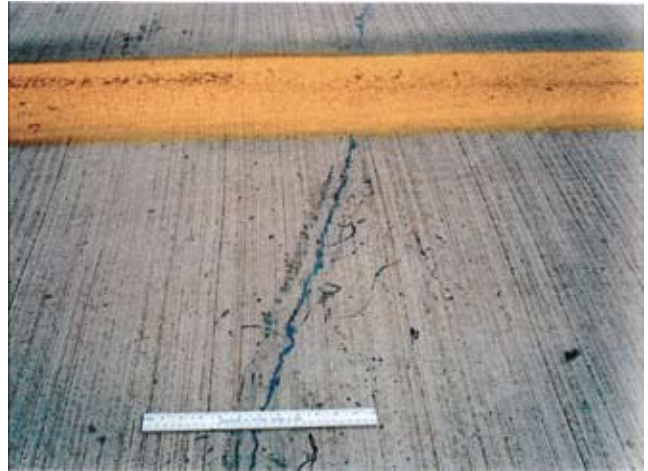
Above: An epoxied crack, 10 years after repair, is totally closed; there is no spalling. Non-destructive deflection tests determined that it functions exactly like the uncracked areas of the pavement.
