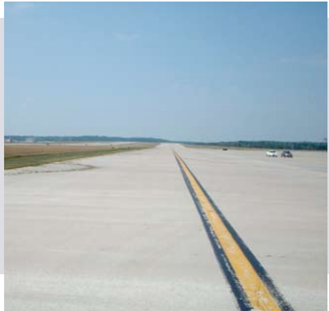
An inspection team reported that, even after 10 years of heavy use, the Type K post-tensioned pavement appeared in almost new condition.
