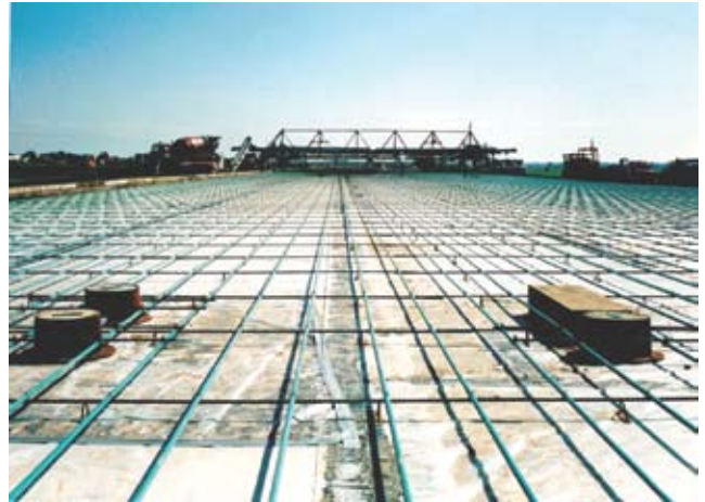
The 0.6-inch-diameter post-tensioning tendons were slightly stronger than standard 0.5-inch tendons. In the background, the bridge-deck paver is ready to go.
