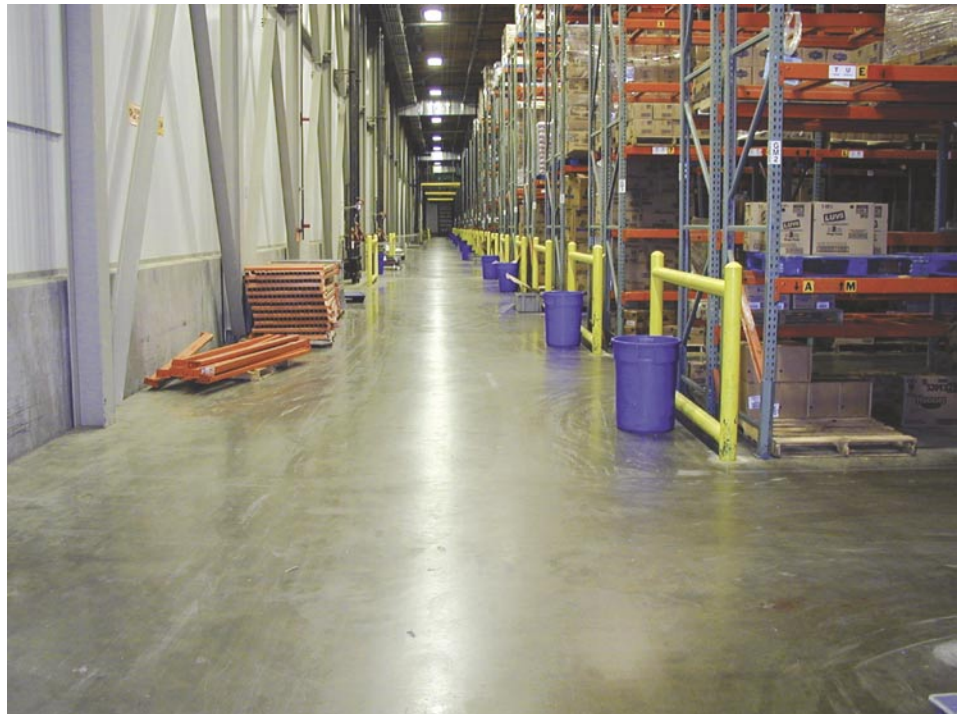
A shrinkage-compensating concrete floor performs beautifully after 10 years of use in an Albertsons distribution center near Phoenix, Arizona.
