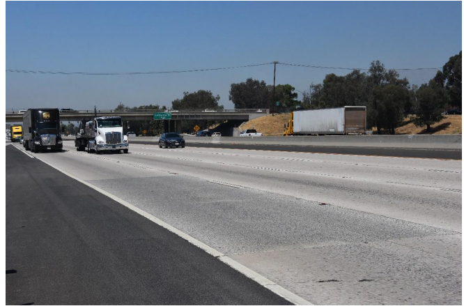
Fig. 3. Highway I-10 EB direction (PM 0-39), near San Bernardino showing two 14-year old RSC slabs in Lane #4 (outer lane).
