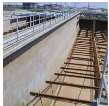
Fig. 2 – Jonathon W. Rogers Water Treatment Plant.
