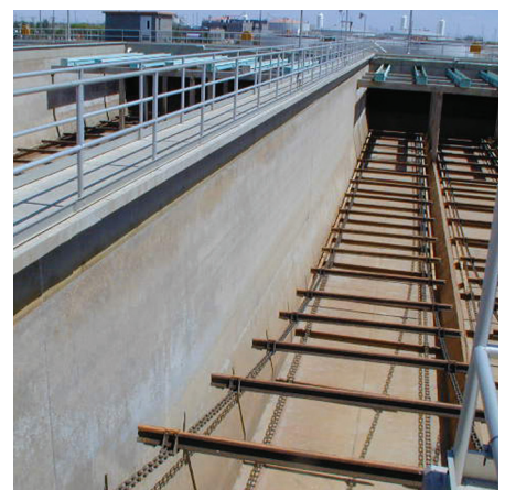
Fig. 2 – Jonathon W. Rogers Water Treatment Plant.
