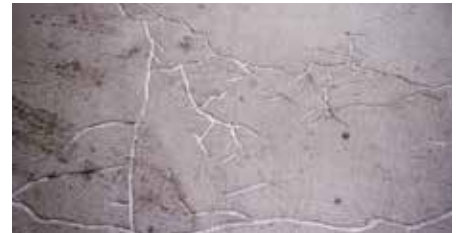
Fig. 9 – 70,000 ft of cracking in Level 1 of the original structure was routed out and sealed to eliminate water infiltrating the slabs or leaking through onto cars on Level 0 below.
