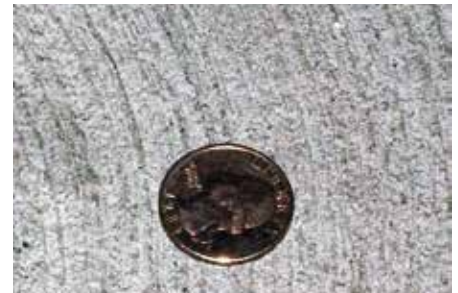
Fig. 10 – After nine years of heavy traffic, the swirled trowel-patterns on the Type K concrete on Level 2 are still crisp and looking new, due to the material’s superior abrasion resistance.
