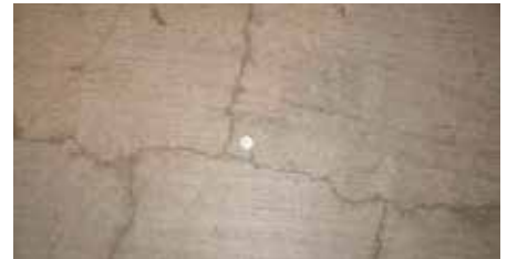
Fig. 8 – When the original structure was built, the slabs made with portland cement concrete exhibited drying-shrinkage cracking before the concrete was strong enough for post-tensioning.
