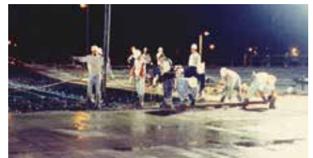
Fig. 12 – Type K concrete was placed at night to accommodate airport traffic regulations and to protect the fresh concrete from excessive summer heat.
