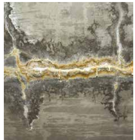
Fig. 6 – Cracks in the Level 1 deck of the original structure as seen from the underside. Water leaking through the cracks carried lime from the interior of the conventional concrete, depositing disfiguring efflorescence and dripping onto cars on Level 0.
