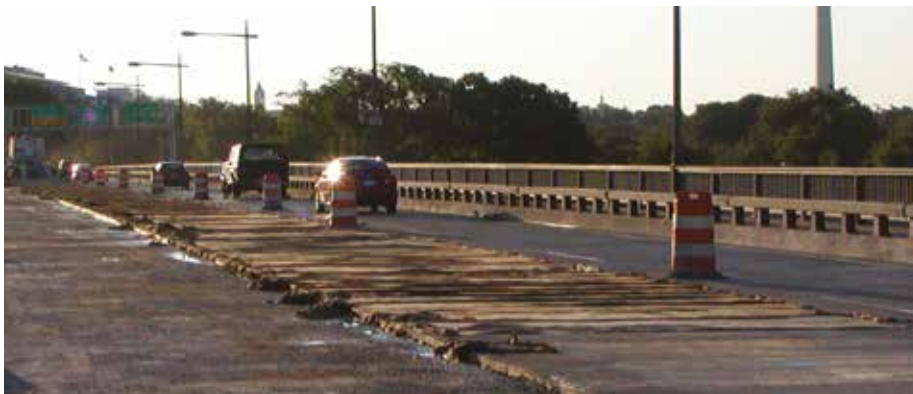
Traffic is maintained as workers repair the concrete deck of the Theodore Roosevelt Bridge in Washington, D.C. Photo: CTS Cement Manufacturing Corp.
