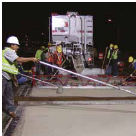
Bridge deck overlays placed at night using early strength cement can minimize inconvenience to motorists. Photo: CTS Cement Manufacturing Corp.
