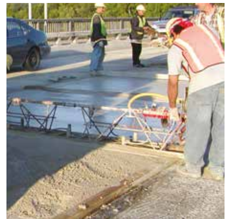
In 1997, the Virginia Transportation Research Council together with the Virginia Department of Transportation placed overlays on two bridges using a very early strength cement. Photo: CTS Cement Manufacturing Corp.
