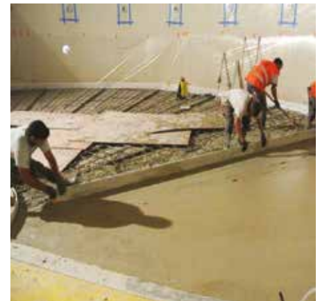
Swiss Factory Setting: The full-depth repair of the 2,150-square-foot floor required the additive Concrete Pharmacy SET Control, which slows the set time of cement, because temperatures both inside and outside of the building were high on the day of the pour.
