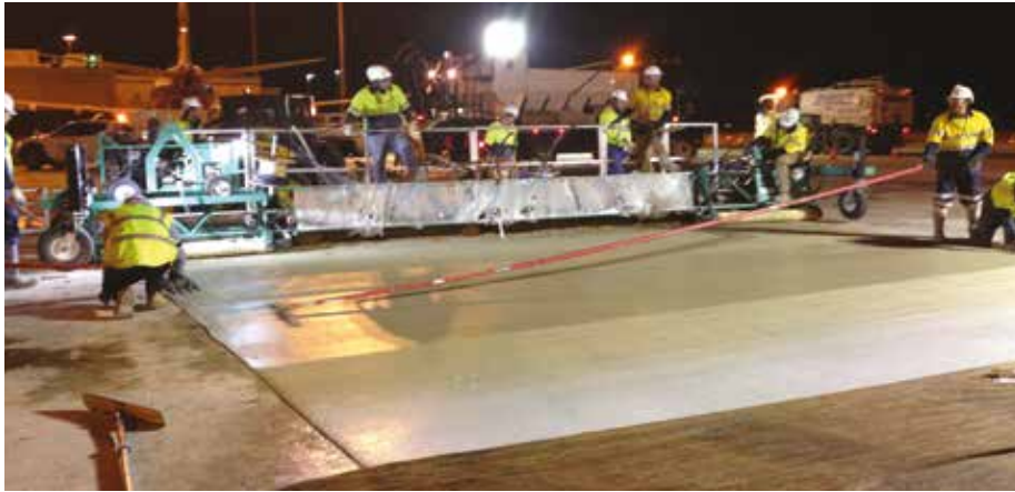
SYDNEY INTERNATIONAL AIRPORT: They only had six hours working time and replaced pavements needed to be strong enough by 5 a.m. to handle aircraft traffic loading.
