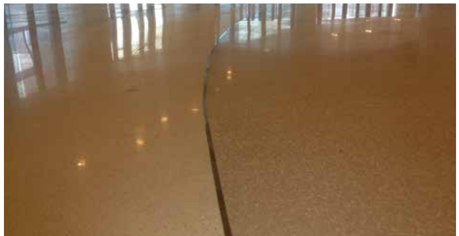
SUZHOU, EASTERN CHINA: By using TRU Self-Leveling they were able to achieve seamless joints and incorporate multiple colors in swirled patterns across the floor's surface.
