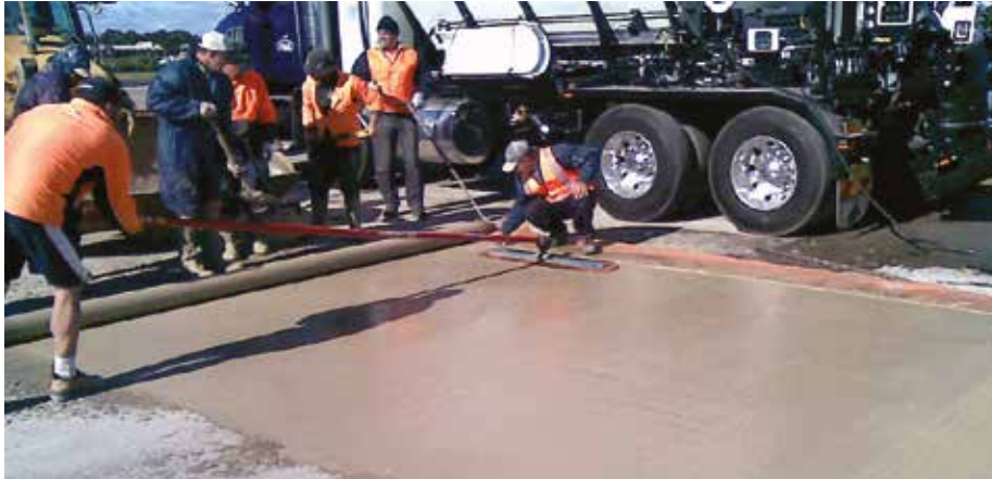
To minimize disruption to air traffic and scheduling at this heavily traveled Sydney International Airport, the crew worked only at night to repair damaged slabs. They only had six hours working time and replaced pavements needed to be strong enough by 5 a.m. to handle aircraft traffic loading.
