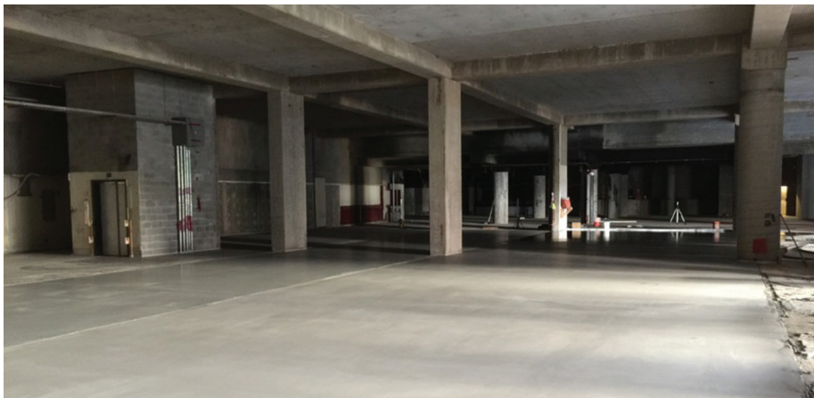
Nordstrom specified Rapid Set® Products for the overlay, which included LevelFlor® self-leveling underlayment, TXP™ Epoxy Primer and TRU® Self-Leveling topping. CTS RAPID SET
