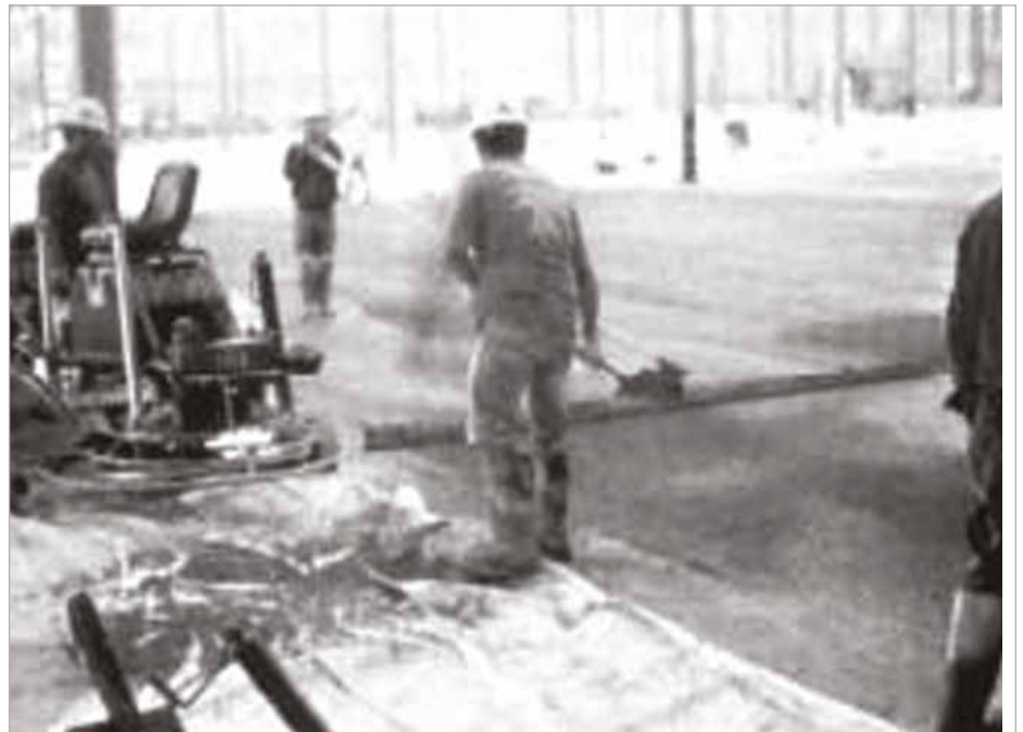
Fig. 8 – SCC floor finishing and application of field-mixed trap rock hardener. Note: 12 ft (3.7 m) long highway straight-edge assisted in attaining high (thus good) FF (flatness) numbers. Note: riding double-towel machine at left, which also helped in attaining a very flat floor when “pizza pans” were attached to the blades.
