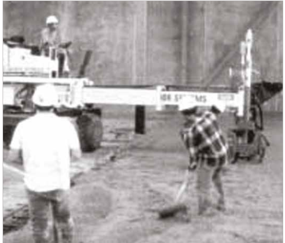
Fig. 7 – Laser screed striking off and consolidating concrete placement by means of telescoping boom with elevation controlled by laser. Laser screed assisted in attaining high (thus good) FL (levelness) numbers. Note: optimized concrete mixture that appears harsh and “stony” but is actually extremely workable and finishable.
