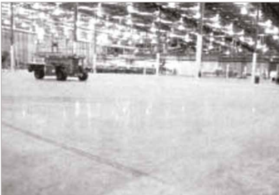
Fig. 10 – SCC finished floor with joints as far apart as 125 ft. (38 m). Note: steel angle armored construction joint (extending from center to left of photo) in lift truck traffic aisle; tight floor joints exhibiting very little shrinkage, considering large slab panels.
