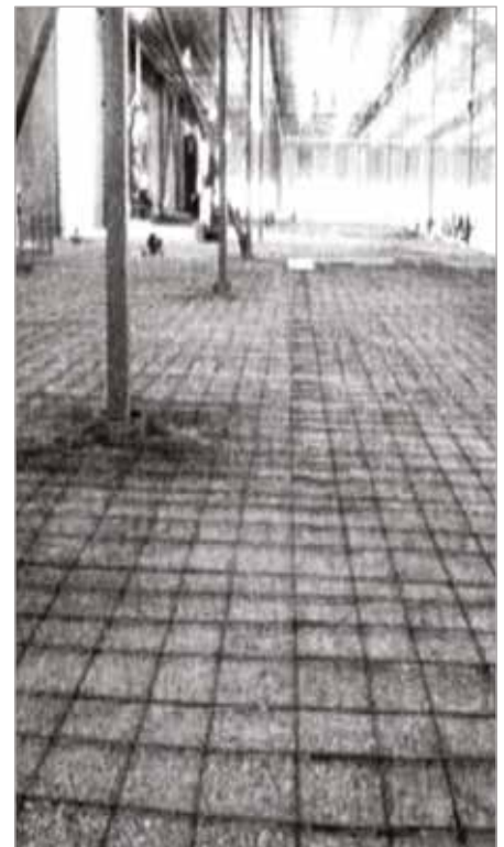
Fig. 2 – SCC floor panel almost ready for concrete placement. Note: 125 ft (38 m) joint spacing with no intermediate joints. Note: reinforcing bar mat lying on level, stiff low-friction, granular base material. Concrete trucks and laser screed will drive over reinforcing steel, which will be chaired up just behind vehicles.
