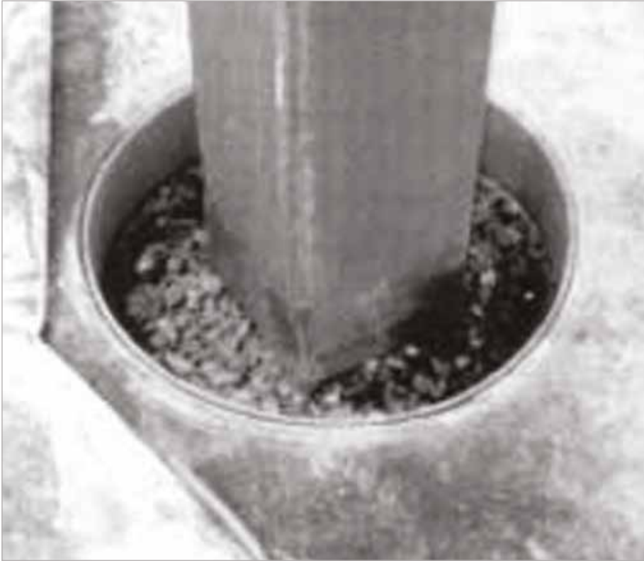
Fig. 9 – Column round isolation section not located at construction joints. Note: soft polyethylene foam isolation joint material (instead of stiff premolded joint filler used for typical PCC floors) to allow for SCC movement; peeled back special curling sheets of white synthetic fiber with white plastic backing.
