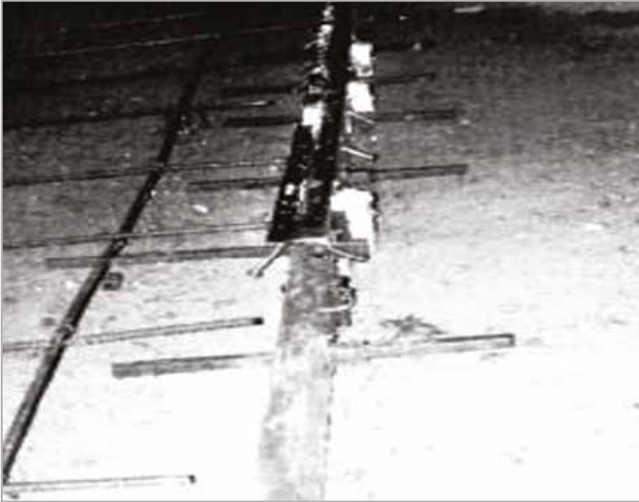
Fig. 3 – Prefabricated system consisting of steel angle armored floor construction joint, edge forms with and without armor angles, reusable dowel holders/aligners (red), etc. Note: No. 4 (12 mm) reinforcing steel at 18 in. (450 mm) on center for proper SCC expansion restraint, not structural purposes.
