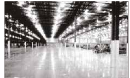
Fig. 11 – Finished slab with as much as 125 ft (38 m) between joints. Note: very straight column reflections, indicating a very flat floor; shiny, burnished floor surface (there is no coating or sealer causing the shine); armored angle construction joint in foreground.
