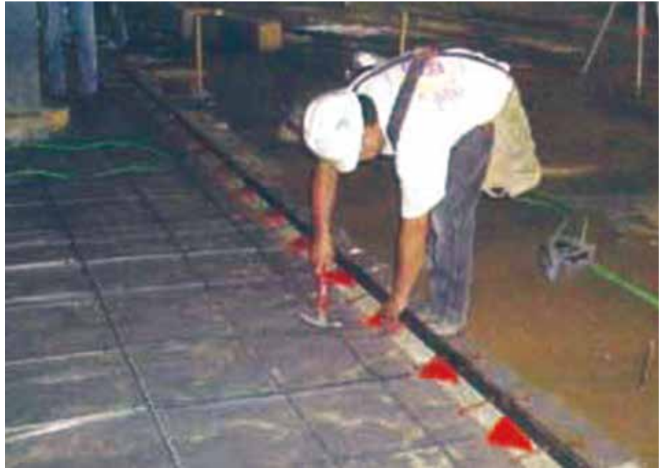
Fig. 3 – The plate dowel pocket former is nailed to the form prior to casting the first slab.
