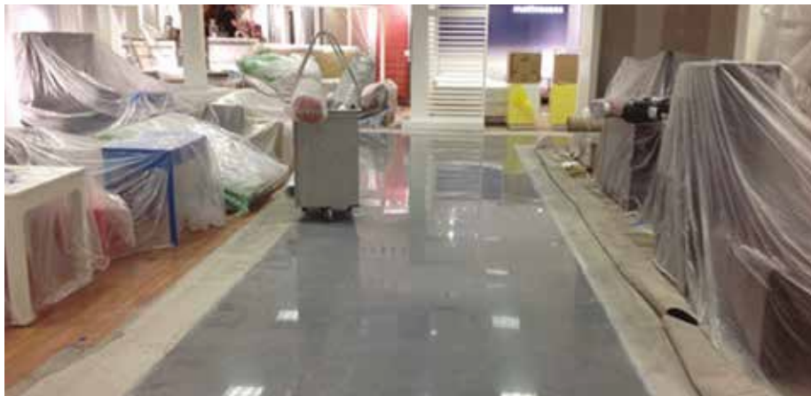
Fig 1 - Each night, the merchandise is covered before work can begin on the "streets" in this JCPenney store at West Towne Mall in Madison, Wis. This particular job features CTS Cement's Rapid Set TRU overlay.
