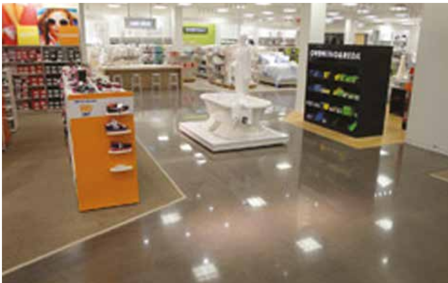
Fig 6 - In this stand-alone store in Canton, Mich., the contractor polished the existing underlayment, but all the joints had to be rebuilt with Rapid Set TRU. It was a massive repair project.
