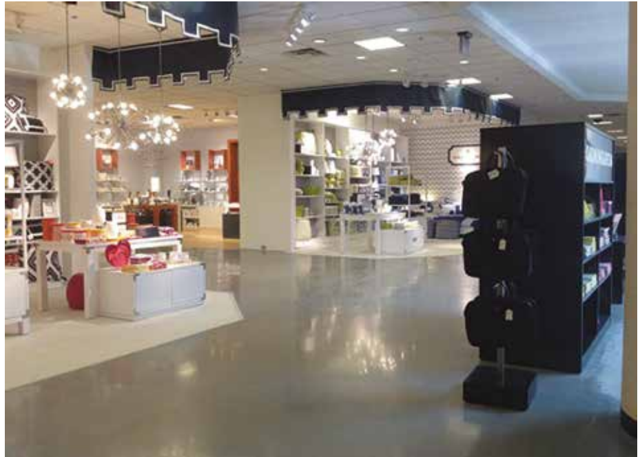
Fig 3 - Each night, the merchandise is covered before work can begin on the "streets" in this JCPenney store at West Towne Mall in Madison, Wis. This particular job features CTS Cement's Rapid Set TRU overlay.
