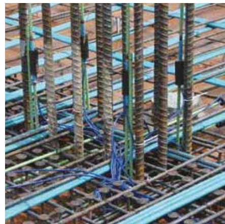
Fig. 5: Vibrating wire strain gauges (black) were welded to epoxy-coated reinforcing bars (green) and connected to a data logger via cables (dark blue). Also visible: post-tensioning strand sheathing (light blue) and headed stud shear reinforcement
