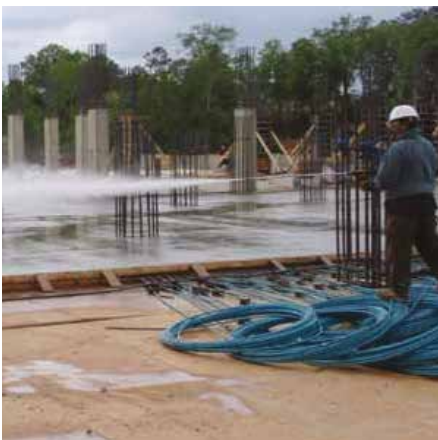
Fig. 4: For the elevated slabs in the garage levels, fogging was started immediately after concrete placement
