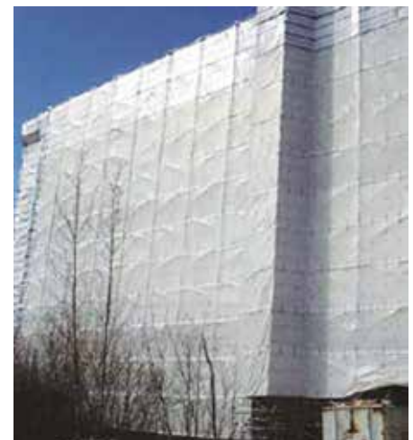
Fig 2 - This eight-story Marriott Hotel project was plastered during the winter in Bellevue, Washington. Due to near-freezing conditions and the heavy rain common to the region, it was tented to protect both plaster and plasterers. Rapid-setting plaster was used, so overnight heating was not necessary.
