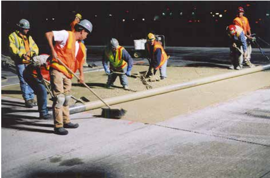
Figure 6. The Seattle-Tacoma international Airport replaced 18-inch thick runway and taxiway slab sections with RHCC during airline downtime (late night and early morning), opening the replaced sections to air traffic only 4 hours after placement. Flexural strength at 4 hours was as high as 800 psi, exceeding the specified flexural strength of 550 psi required for opening to traffic. Laboratory fatigue testing of the concrete with up to 4 million load cycles indicated a probable service life of 87 years.
