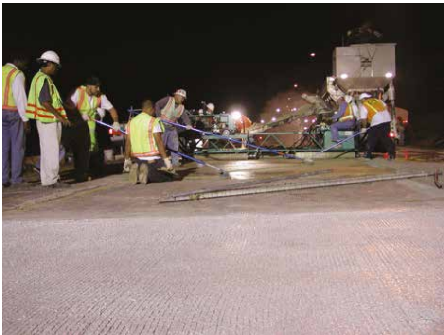
Figure 8. Using latex modified RHCC, the Virginia DOT put down bridge-deck overlays in record time, starting work each night at 9 p.m. and permitting traffic on the new overlay at 5 a.m. the next day. "Because of the reduced cost of traffic control, compared with that incurred with other overlays, the [latex-modified RHCC] overlay is more economical," says Michael M. Sprinkel of the Virginia Transportation Research Council. "It can reduce the cost of hydraulic cement-concrete overlays approximately 25%, and it can minimize the inconvenience of overlay construction to the traveling public."
