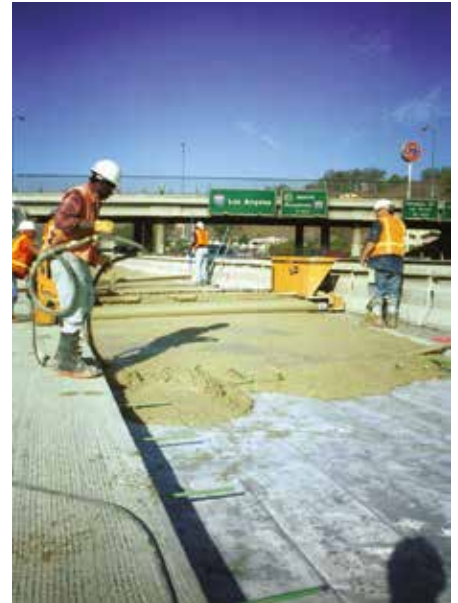
Figure 7. Caltrans removed and replaced 2 lane miles of Interstate 10 near Pomona using RHCC. On a Friday night at 10 p.m., Caltrans shut down two of four East bound lanes in a 3-mile section of the freeway. By 5 a.m. the following Monday morning, the road was reopened.
