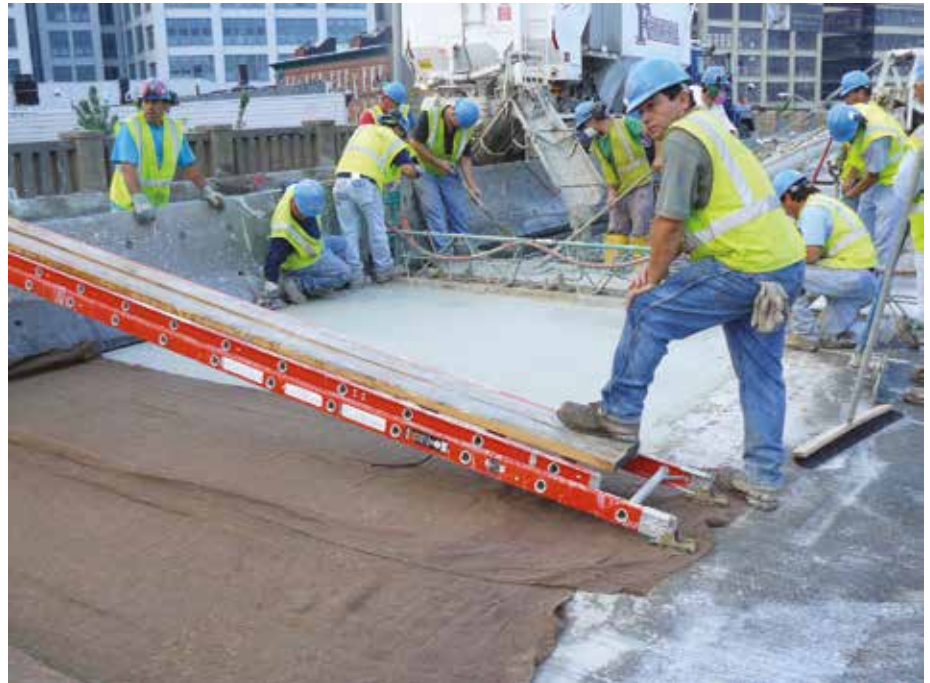
Figure 10. In Chicago, the city's transportation department decided to minimize traffic interruption by using latex-modified RHCC this summer on the 1-90 Skyway Bridge rehabilitation project. Crews removed and replaced 9 cubic yards of concrete each night, with RHCC placement starting at about 2 a.m. so they could open repaired sections to traffic by 6 a.m.
