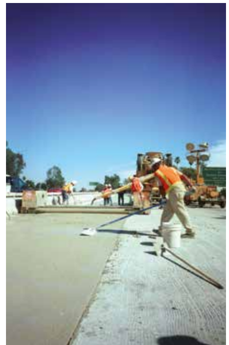
Figure 9. During the intervening 55 hours, Caltrans crews removed the old 9-inch thick pavement from 2 miles of roadway and replaced it with RHCC concrete, which achieved a flexural strength of 445 psi in 4 hours.
