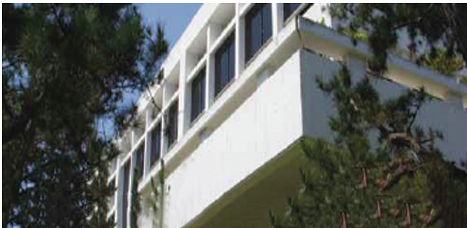
Fig. 5 – Building M5, southeast corner showing dramatic cantilevered post-tensioned beams at Plaza Level. Courtesy of Phillip Yee of Northrop-Grumman.
