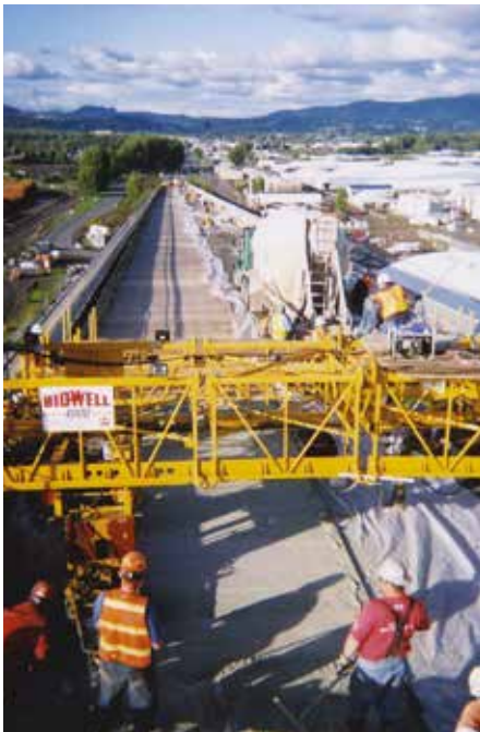
CSA cement was used for the overlay of the 79-year-old Lewis and Clark Bridge over the Columbia River running between Washington and Oregon..
