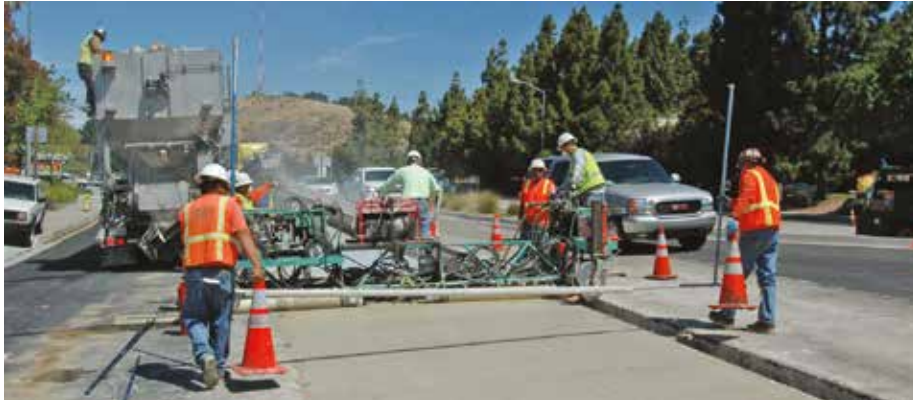
Panel replacement work on Highway 1 with rapid-setting cement in San Luis Obispo, California.
