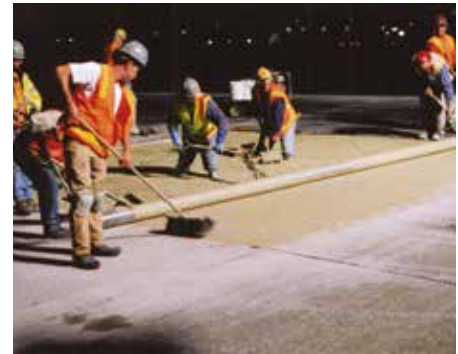
The Seattle-Tacoma (Sea-Tac) runway mix design is a seven-sack CSA concrete tested at the University of Oklahoma to have a lifecycle of more than 80 years.
