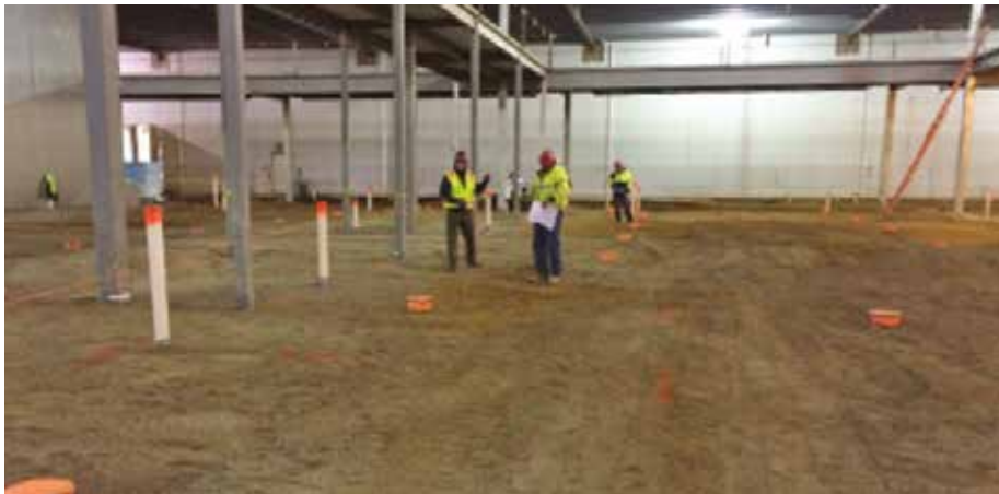
Fig. 1 – One of the major concerns on the project was the extensive plumbing running throughout the floors with a potential for reflective cracking along the pipe placements. Photo Credit: CRT Concrete Consulting.
