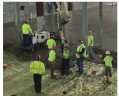
Fig. 3 – After much consideration the contractor chose to utilize a Somero S-840 Laser Screed® machine equipped with the Somero 3-D Profiler System®. The S-840 offered the proper screed head width and was also equipped with a 3D blade to fine-grade the sub-base to accurately control concrete thickness and yield. Photo Credit: CRT Concrete Consulting.
