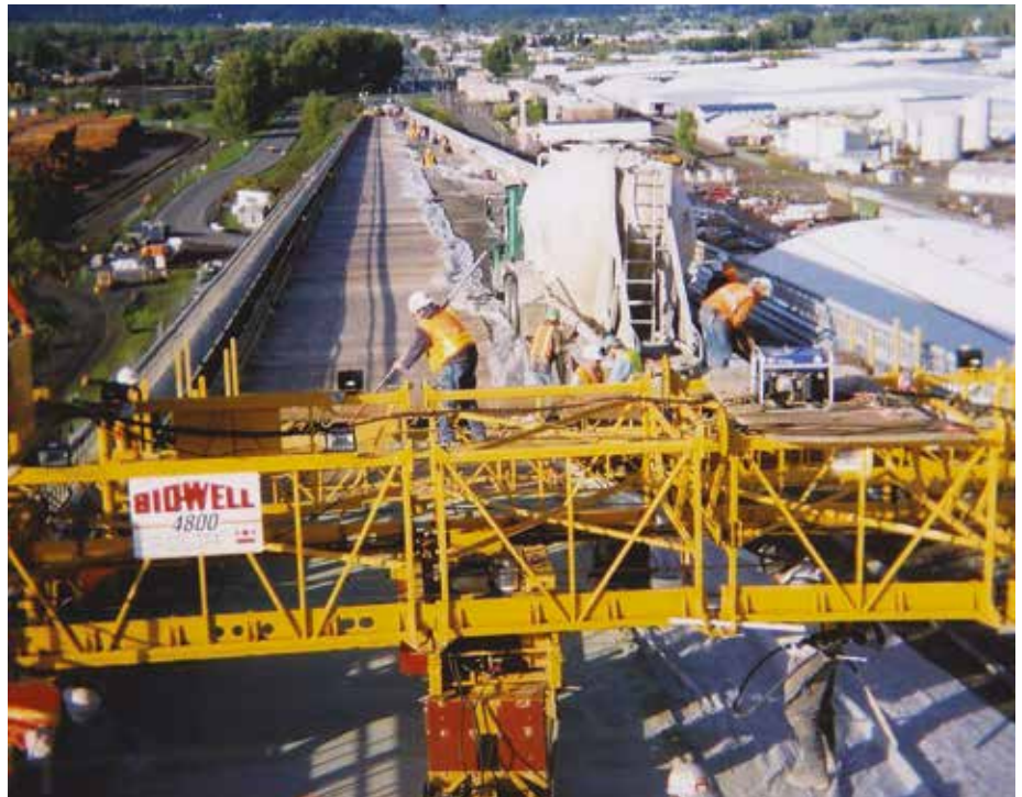
Rapid Set® cement is being used for the overlay of the 79-year-old Lewis and Clark Bridge over the Columbia River between Washington and Oregon.
