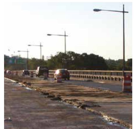
The Theodore Roosevelt Bridge in Washington, D.C. is being repaired with Rapid Set® latex modified concrete. Photos: CTS Cement Manufacturing Corp.
