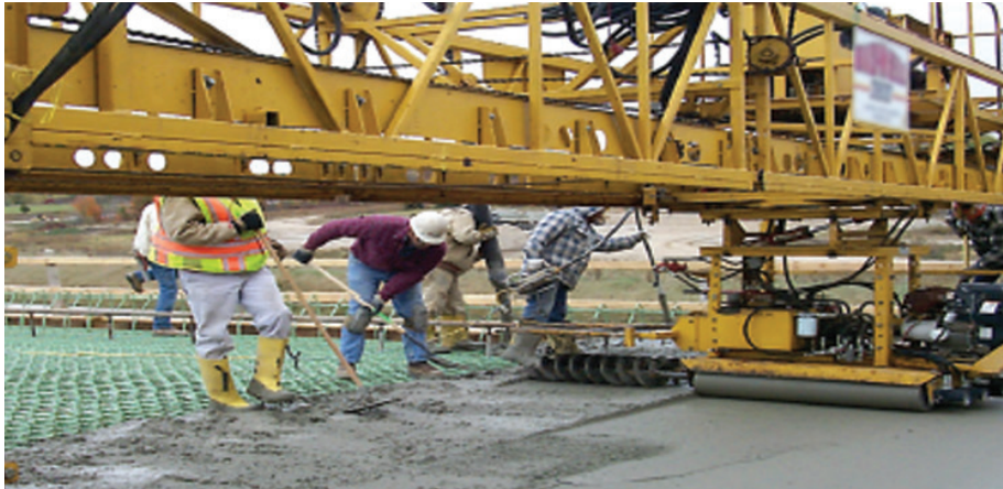
Fig. 1 – Crews use rapid-setting cement for the deck overlay of the M6 Beltway project in Grand Rapids, Mich.
