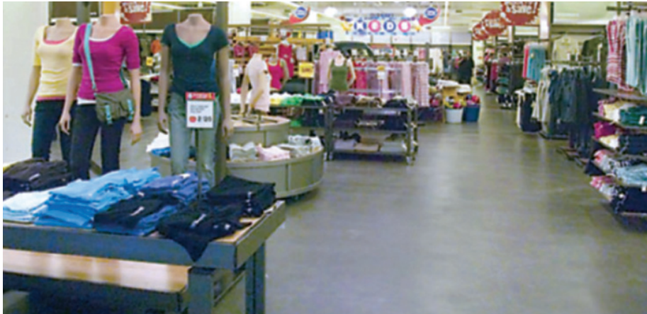
Fig. 1 – Type K cement was used to produce a crack-free concrete floor at an Old Navy store in Portland, Oregon. The space's previous floor had failed due to cracking. Based on this experience and unsuccessful refinishing, the owner requested the use of joints in the replacement floor.
