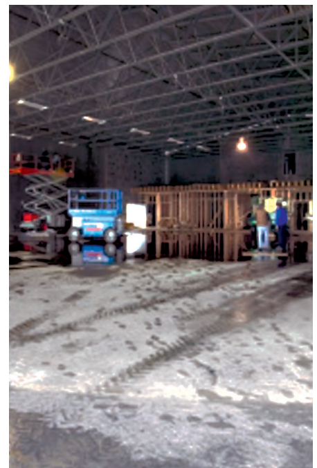
Fig. 2 – Health and safety can be concerns in certain traditional concrete floor applications. For example, heavy forklifts used in warehouses can cause individual slabs to move up and down over time, creating a bump. Shrinkage-compensating concrete does not require the use of control joints.
