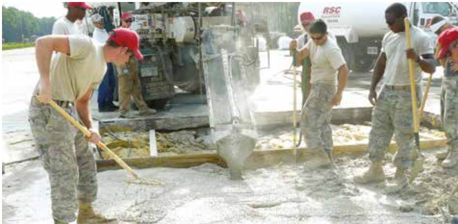
Fig. 1 – Rapid-setting concrete offers technological advances for spall, crack and crater repairs on military airfields.
