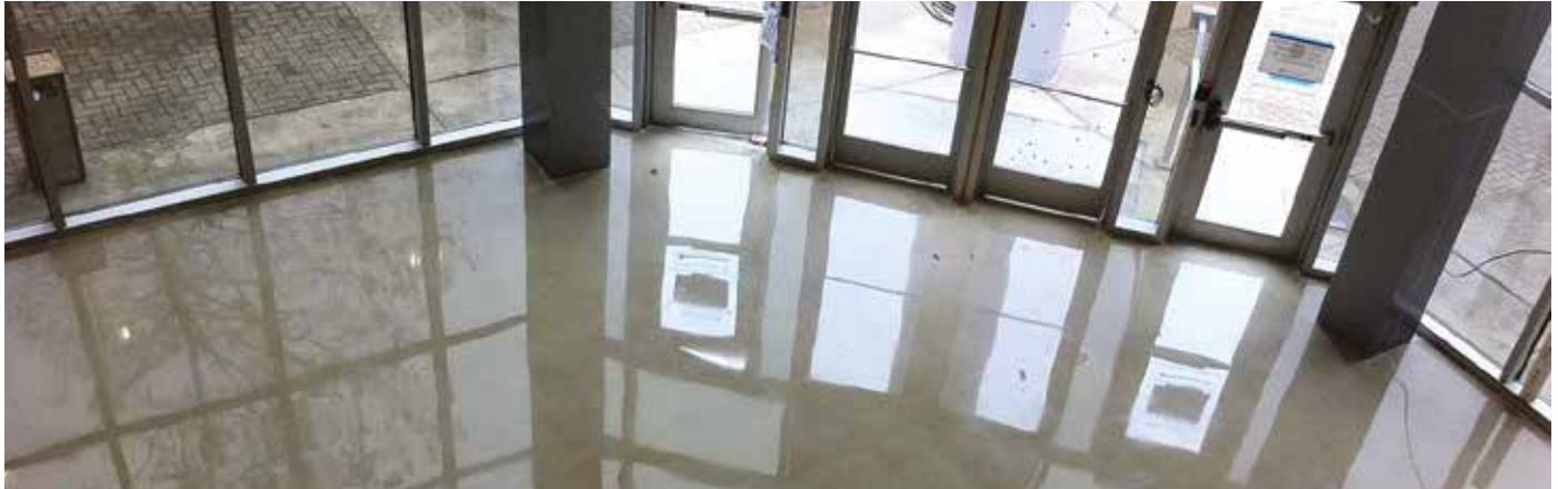
In order to prevent unwanted scratches, the Concrete Visions crew cleaned the floor between each abrasives step to remove any particles left behind from the polishing process.
