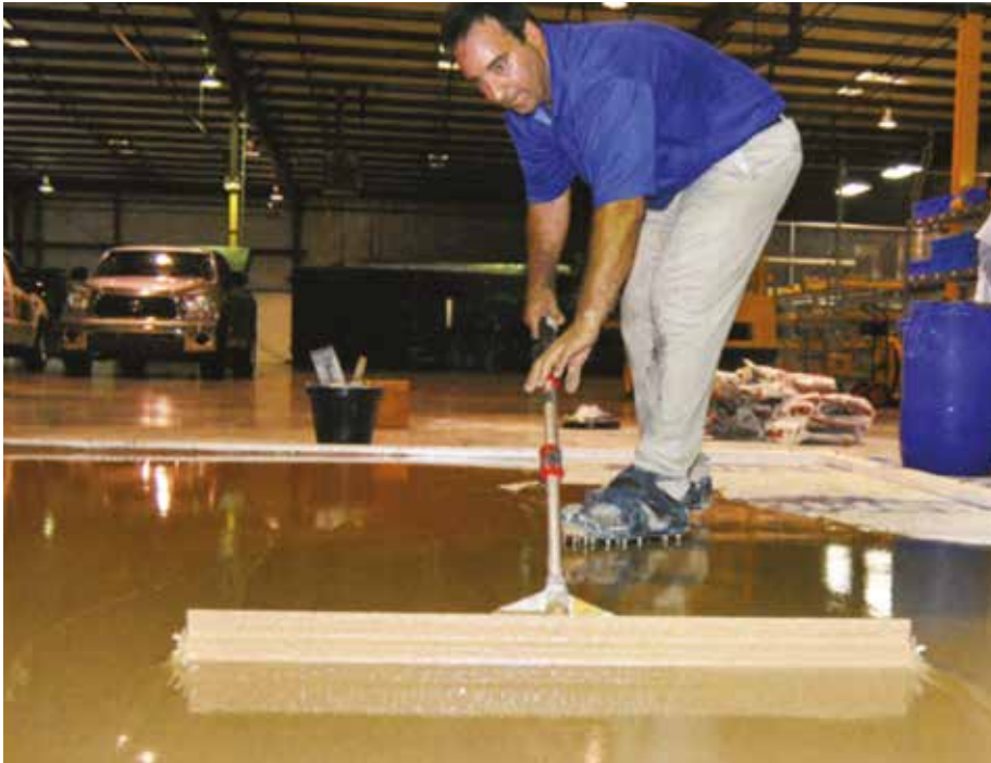
Before the polishing process can begin, an overlayment must be properly raked and spread.
