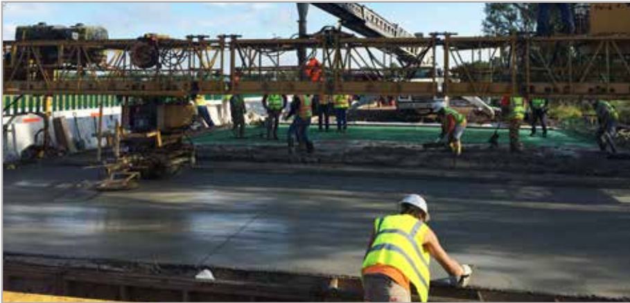
Figure 1 – Stark Excavating places and finishes a Type K cement concrete bridge deck in Peoria, Illinois, over Boyd's Hollow Creek on Route 29. Concrete was supplied by VCNA Prairie.
