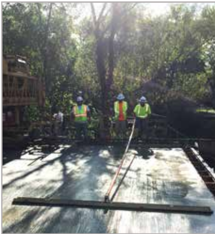
Figure 3 – Workers using a bull float to apply a smooth finish to the Type K cement concrete pavement.
