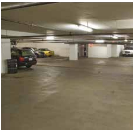
Fig. 3—The floor of the second basement is actually the top surface of the foundation. Forty years after construction, it is crack-free, watertight, and completely dry. The 10 in. (250 mm) thick drop panels of the first basement deck are clearly visible in the ceiling of this photo: they resemble broad soffits surrounding the load-bearing pillars. (Photo by Steven H. Miller, courtesy of CTS Cement Manufacturing.)
