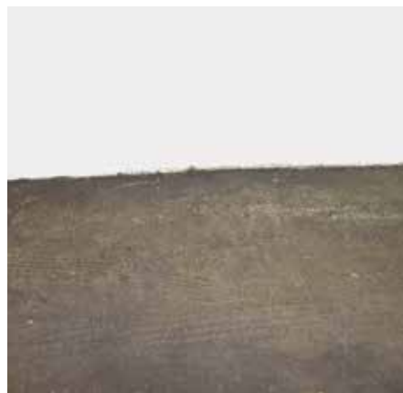
Fig. 4—Even at the meeting point of foundation and basement wall, there is no evidence of cracking or leakage. (Photo by Steven H. Miller, courtesy of CTS Cement Manufacturing.)
