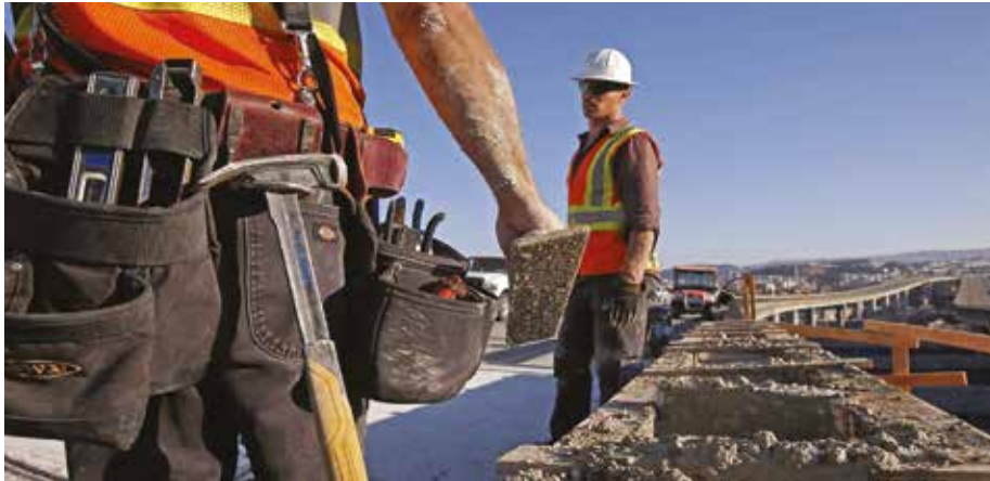
Fig. 1 – The Northbound lanes remain closed as workers continue to put the finishing touches on Interstate 280 freeway project in downtown San Francisco, Calif., on Monday Sept. 1, 2014, to ensure that traffic will be back to normal early Tuesday morning on the Northbound lanes of the elevated freeway between downtown San Francisco and Highway 101, which have been closed since Thursday afternoon while workers replaced two hinges. Photo: Michael Macor, The Chronicle
