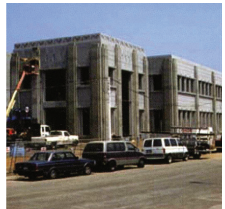
A Santa Fe, California, tilt-up concrete warehouse project comprising a two-story office and a high-bay structure relied on the abilities of new patching compounds to ensure a smooth finish.
