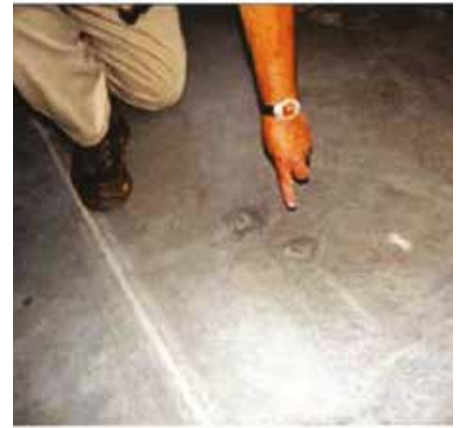
Defects in the floor slab will transfer onto the surface of a tilt-up wall panel—even after attempts have been made to repair the floor. This photo shows a caulked control joint (by foot), patched holes left by fasteners used to install formwork (under finger), and residue from sealant that had been used between formwork and floor slab (across bottom of photo).
