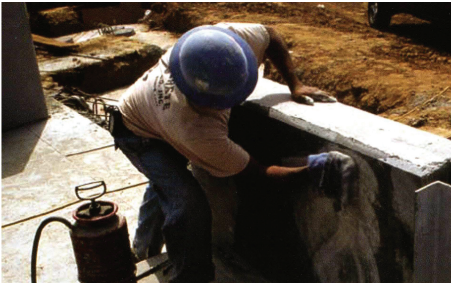
Old methods of sacking and patching required laborious rubbing and meant visual uniformity of results could be difficult. After wetting the wall with a cement slurry, laborers had to rough a silica sand/cement mixture against the wall and rub it into the surface.
