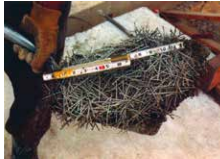
Fig. 7 – Steel fibers 2.5 in. long created tensile forces to hold the slab in compression as Type K cement expanded.
