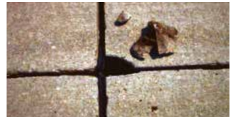
Fig. 9 – Joints in the non-post-tensioned pavement show the spalling typical of 10 years of heavy aircraft traffic and snowplow damage.
