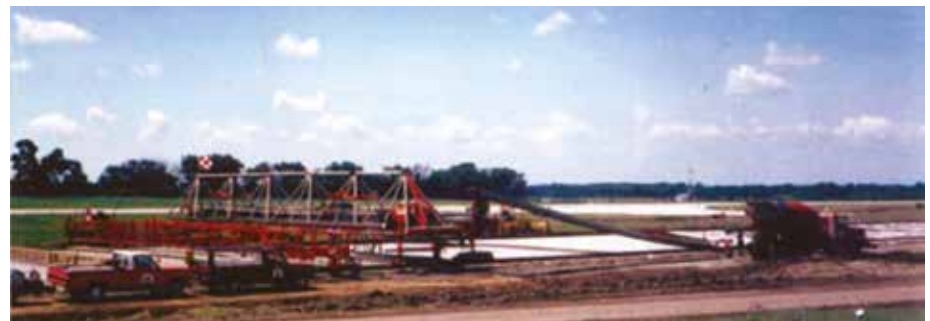
Fig. 4 – The bridge deck paver, an 80-foot truss with conveyor belts, and a truck feeding it concrete.
