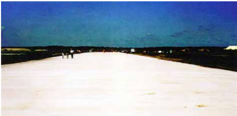
Fig. 1 – The finished 1200 foot slab shortly after pouring, probably the longest unjointed concrete pavement in North America.
