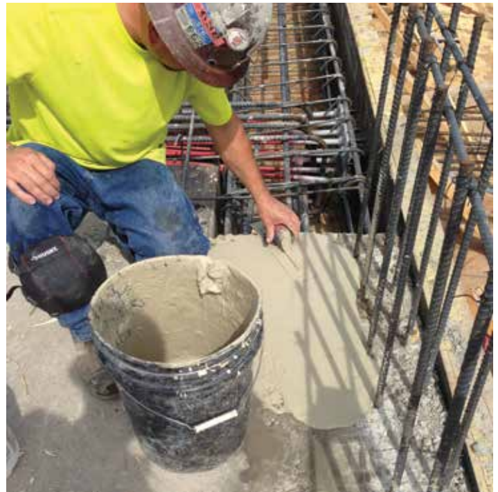
The crew mixes a trial batch to test the color of the mix, to ensure the right amount of the Rapid Set® Dark additive is used to match the repairs to the concrete.
