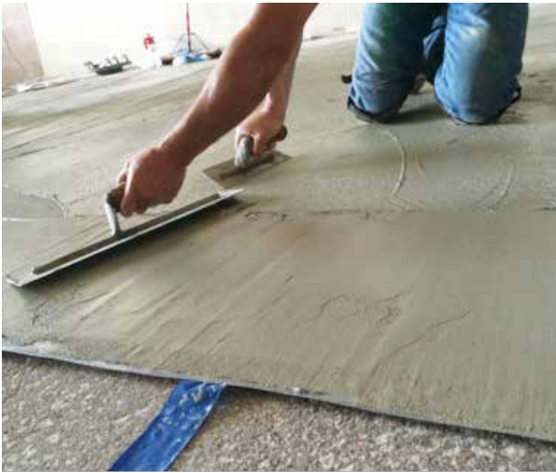
A crew member builds Cement All to the desired thickness of ¼ inch.
