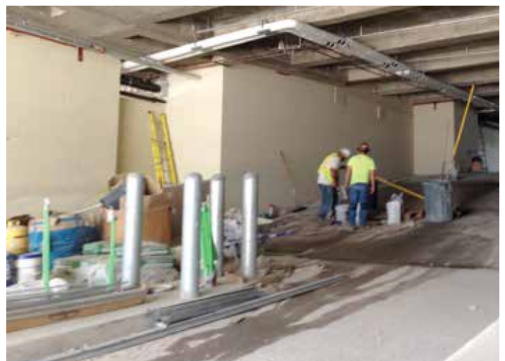
A crew member applies a scrub coat. This method is used to improve adhesion.
