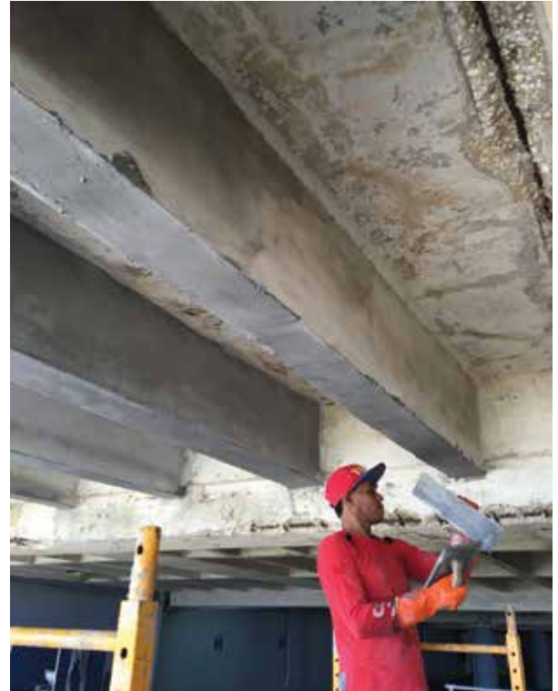
The crew removed the top damaged slabs and replaced it with V/O Repair Mix.
